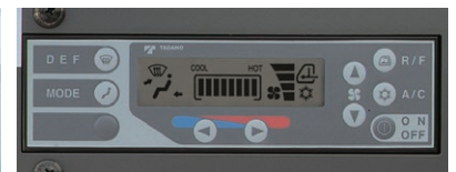
Air conditioning and heating Hot-water heater and air conditioning.
